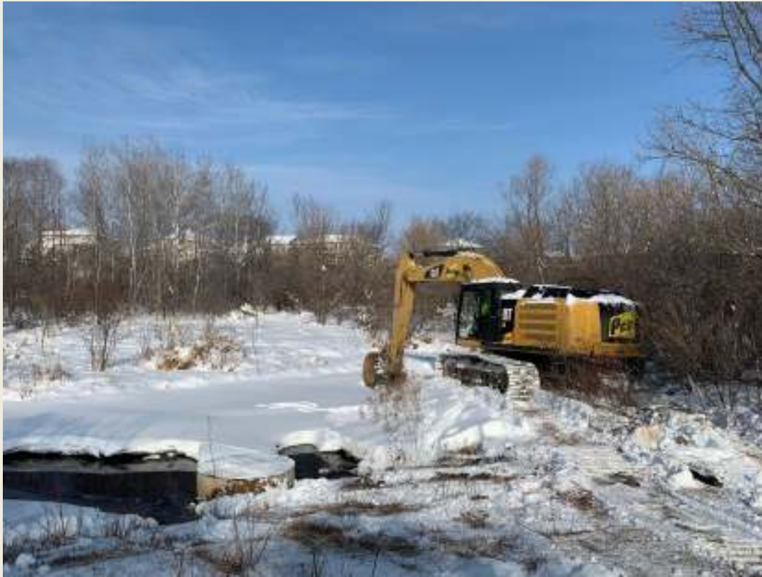
Above: Winter pump harvest pond sediment removal Right: IESF surface aeration
