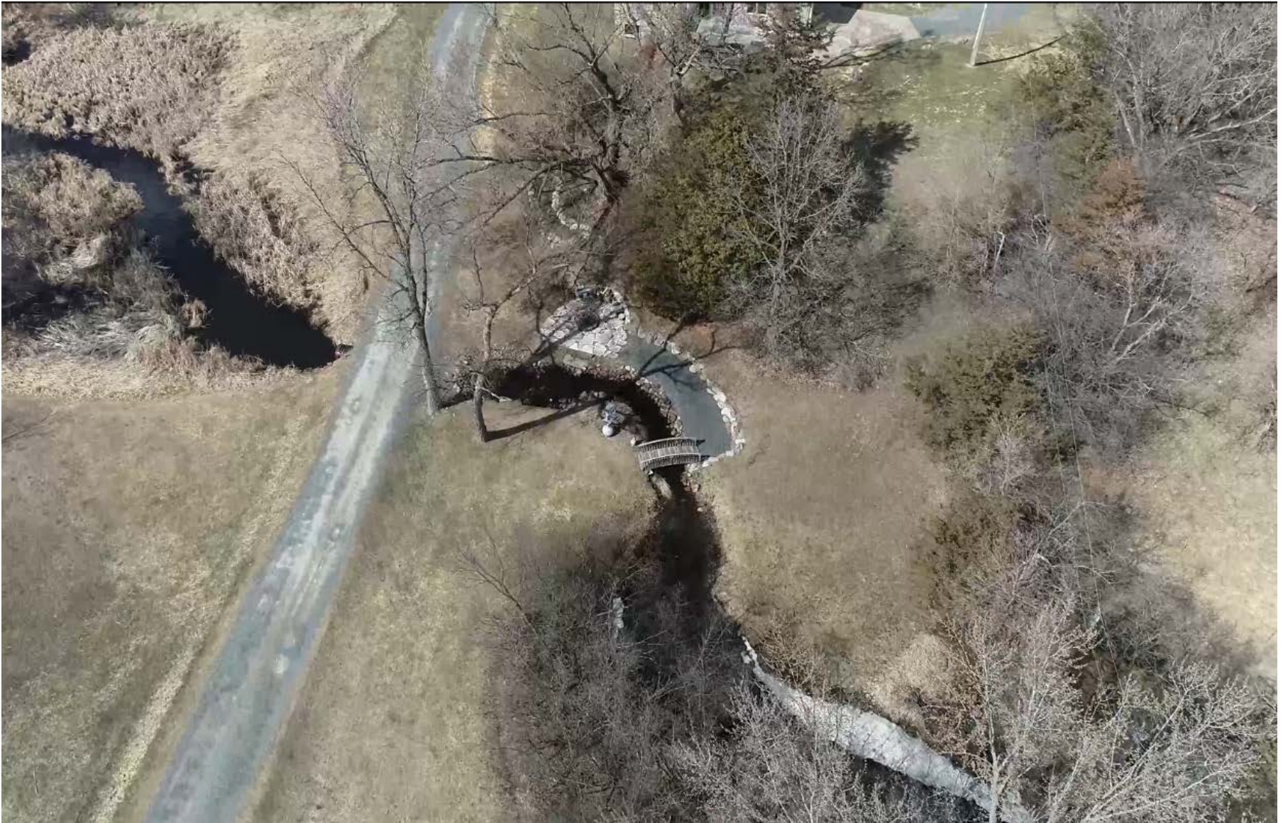
Driveway crossing and small foot bridge over Brown's Creek just upstream of 110 th St
