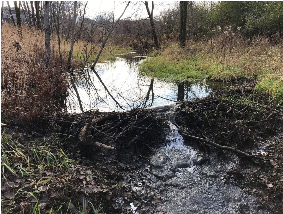
Figure 1. One of three small beaver dams upstream of the wood walk bridge north of the IESF filter.
