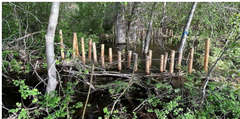
Figure 34: Methow Okanogan Beaver Project BDA installation showing beaver beginning to build upon the BDA that is located near a beaver relocation release site near Twisp, WA. Photo Credit: Jackie Corday.
