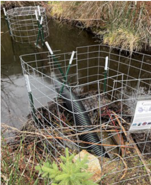
Figure 26: An example fence and pipe device installation. Device designs are site-specific and using the basic design principles, can be adapted for a variety of different waterways by a trained professional. Photo Credit: Elissa Chott.
